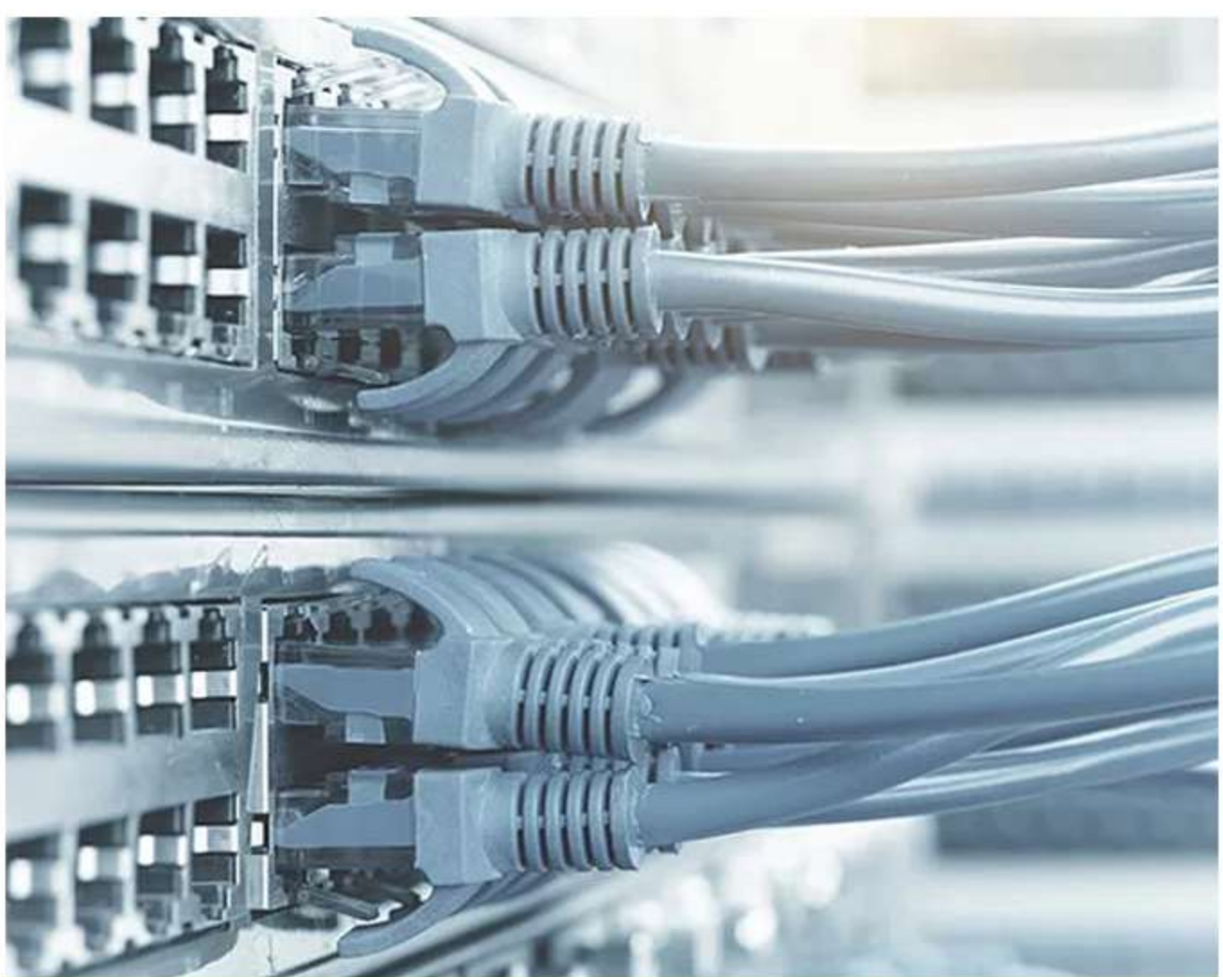
ENTERPRISE STRUCTURE CABLING
